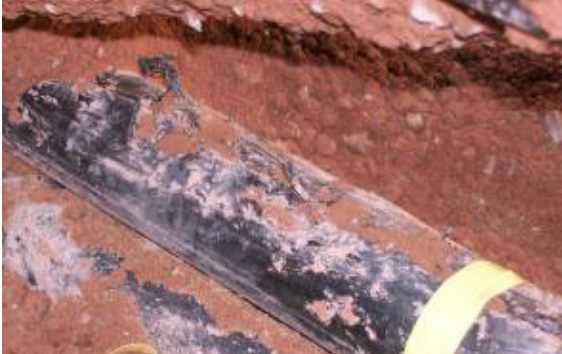
Figure 3. Cable damage missed by a VLF AC withstand and pinpointed with off-line 50/60Hz PD test
