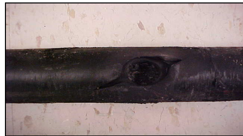
Figure 2. Cable failure prior to off-line 50/60Hz PD test
