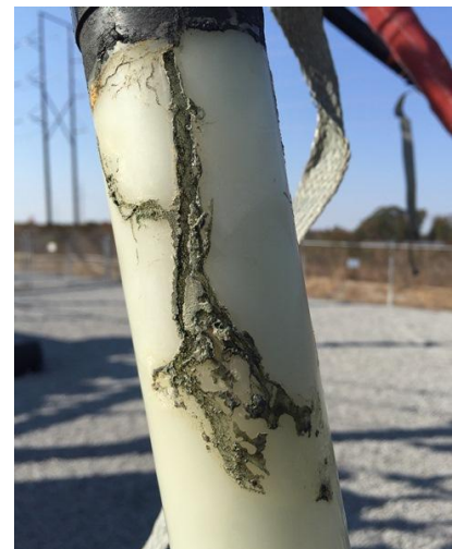
Inside: Installation defects & VLF test damage
