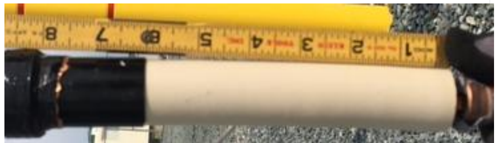
Figure 1: Field dissection revealing incorrect 6-inch semicon (black layer) cutback.
